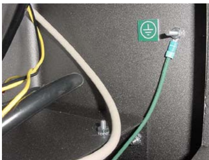
Figure 11 Grounding post in the lower section of tower with cable securely connected.
